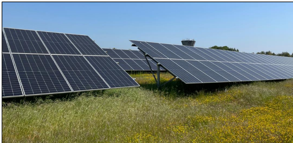
Figure 8.3: Example Side view of PV Arrays
